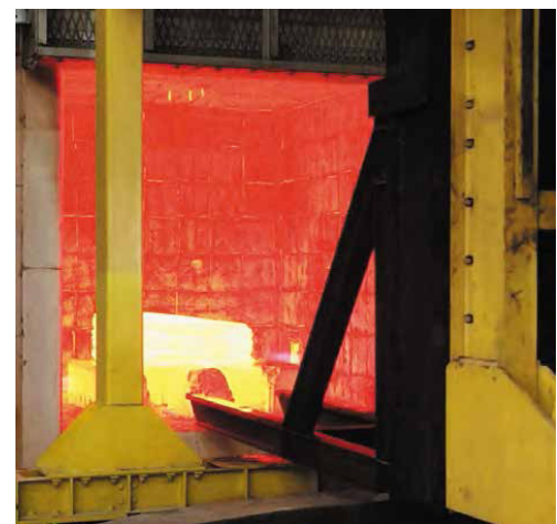
Batch annealing furnace
